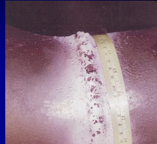
Corrosion in welds
