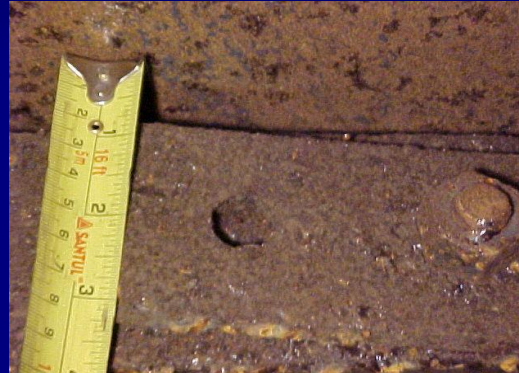
Lack of complete structure
