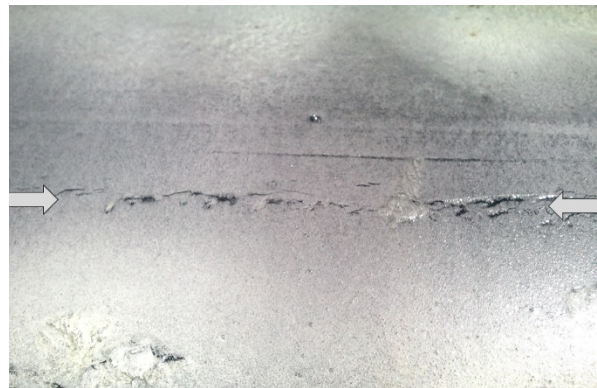
Figure 9: Arrows point to line of contact marks on single side of the ERW weld. Also, linear visual indication showing at centerline of weld. (Courtesy of Riccardelli Consulting Services)
